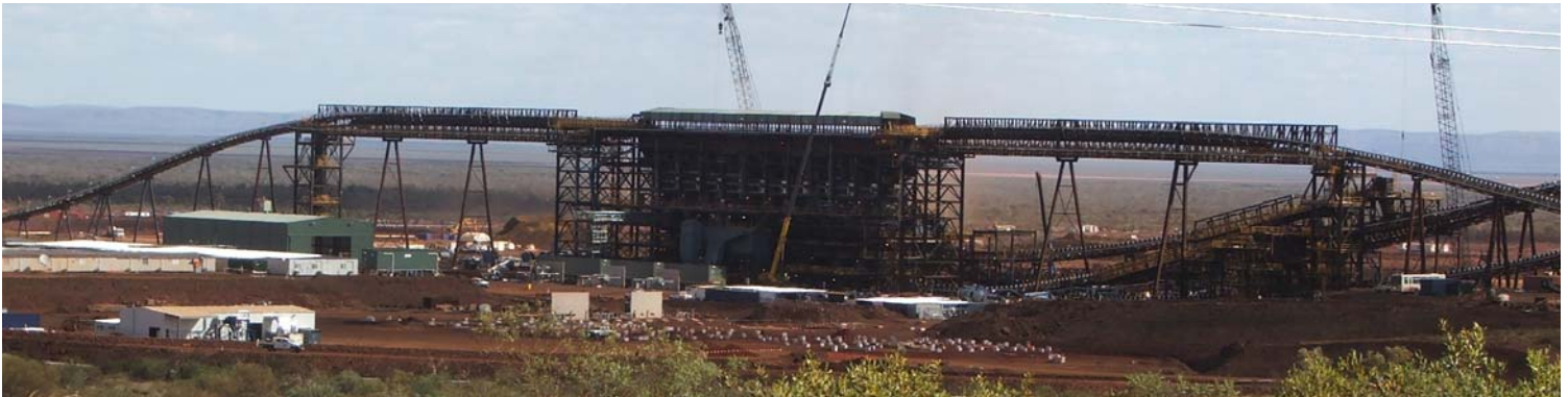
Screening building being commissioned
